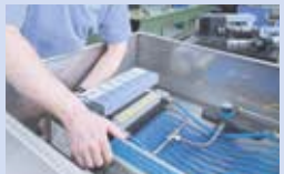
Control cabinets for hazardous locations Page 34
