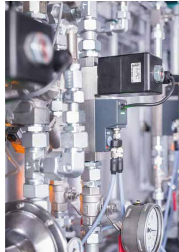
System engineering know-how enables easy start-up of a new roller hearth furnace
