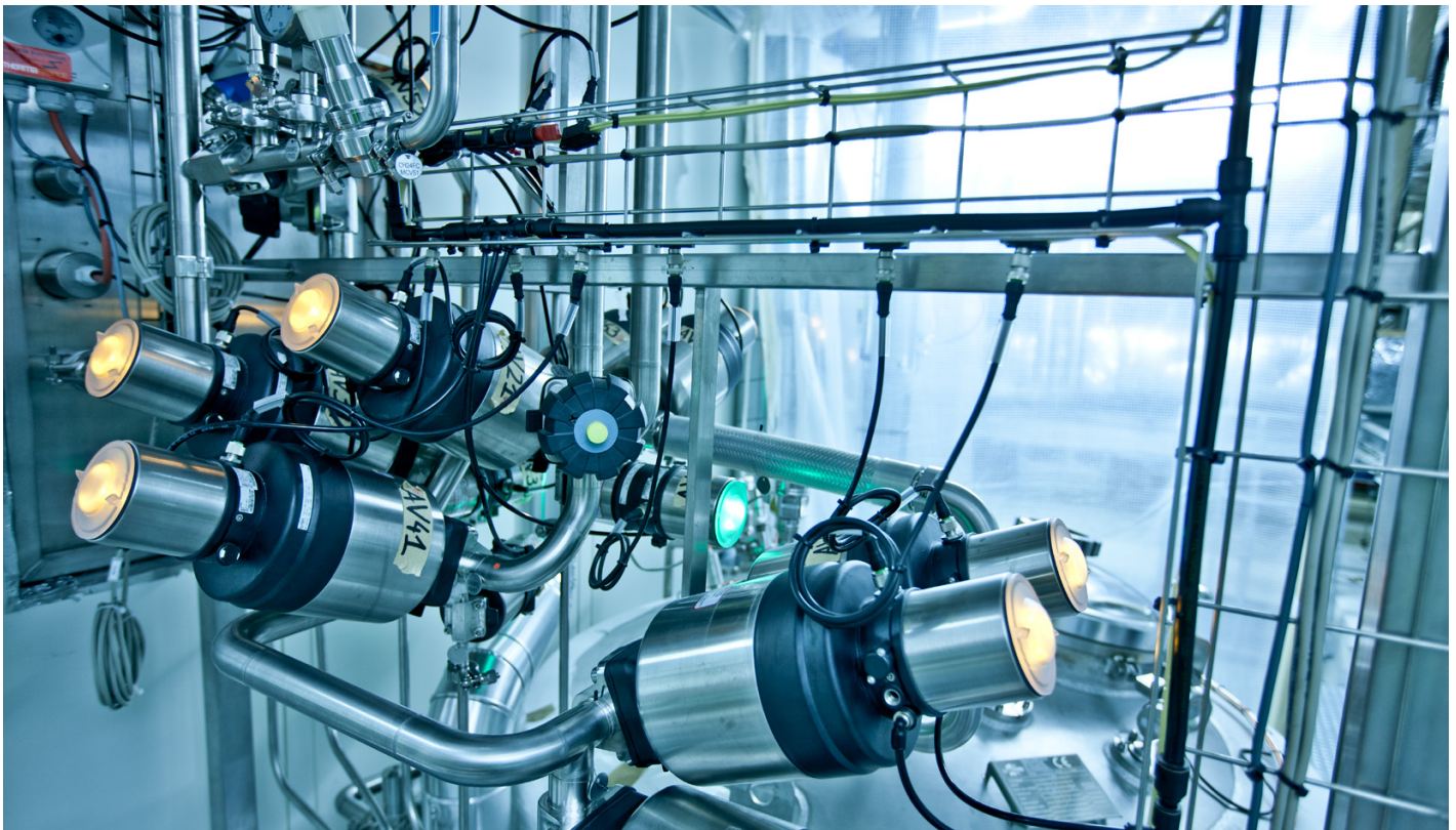
Diaphragm valve type 2103 with control head type 8691 in a clean room at Novo Nordisk
